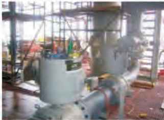
(Floating) Platform - 3 valves with ATC Spring Return Actuators, closely installed on horizontal and vertical mounted valves
